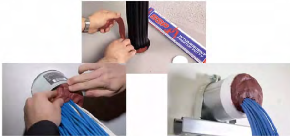
Fire stopped openings
